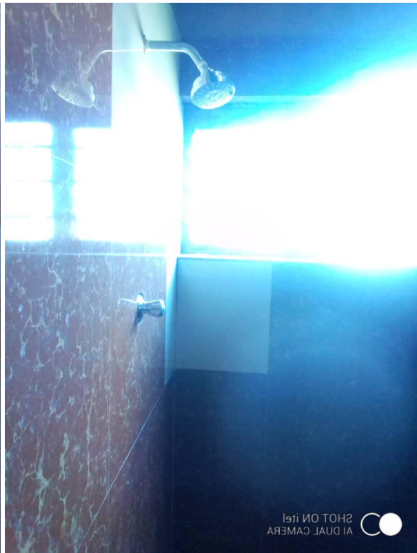
Shower ECO had installed
